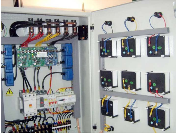
Gambar 14. Panel kontrol ELC (Electronic Load Controller)
