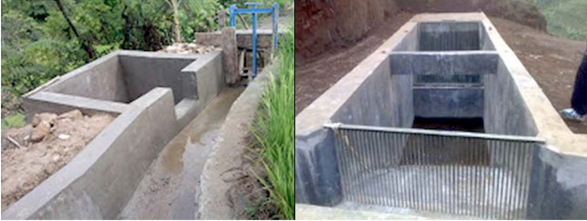
Gambar 7. Saluran Pelimpah (Spillway) dan Kolam Penenang (Forebay)
