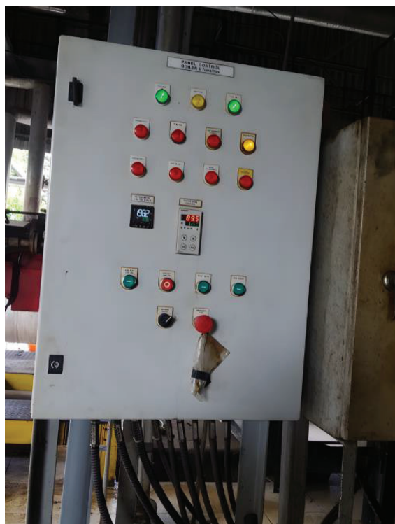
Gambar 2. Panel Kontrol Boiler
