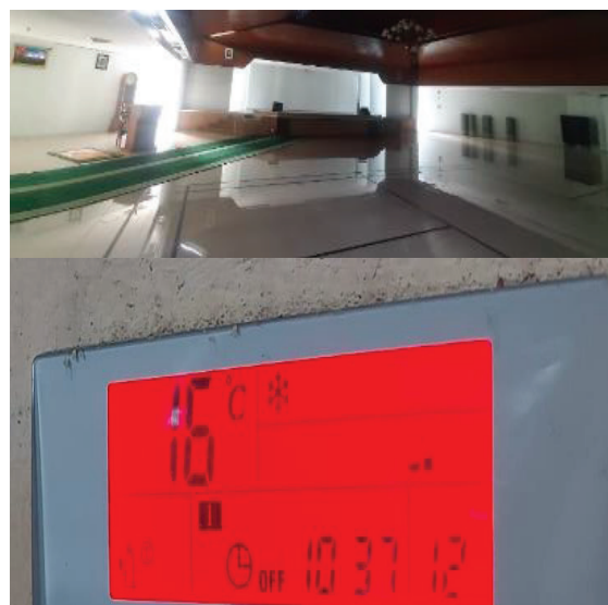
Figure 9. Cooling room activity in 2nd floor but there's no occupation and Temperature from AHU on every floor
