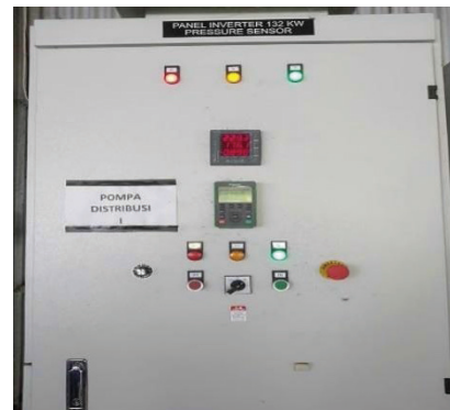
Gambar 4. Panel Sensor Pompa Distribusi I Unit Water Treatment Plant
