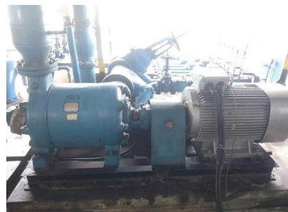
Gambar 3. Pompa Distribusi I Unit Water Treatment Plant
