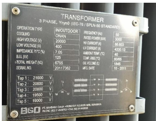
Gambar name plate trafo
